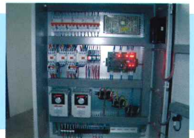
Booster Pump Control Panel
